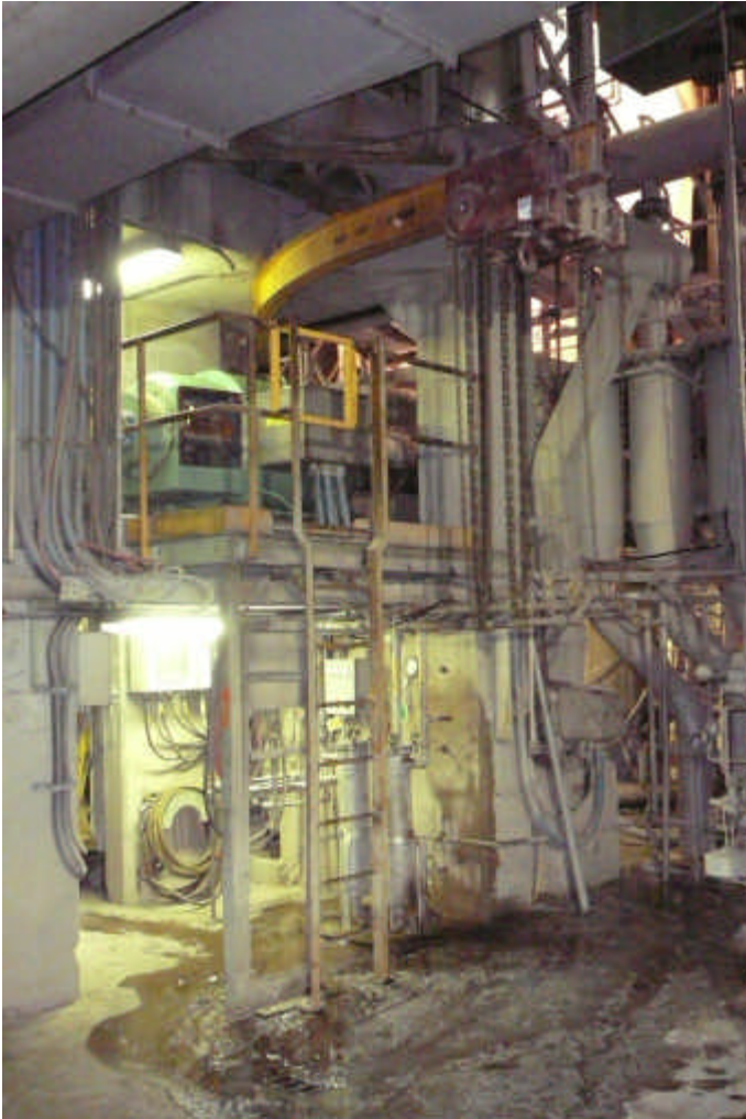
Figure 1 Bottom of pedestal showing intermediate level motor with paper machine to the right
